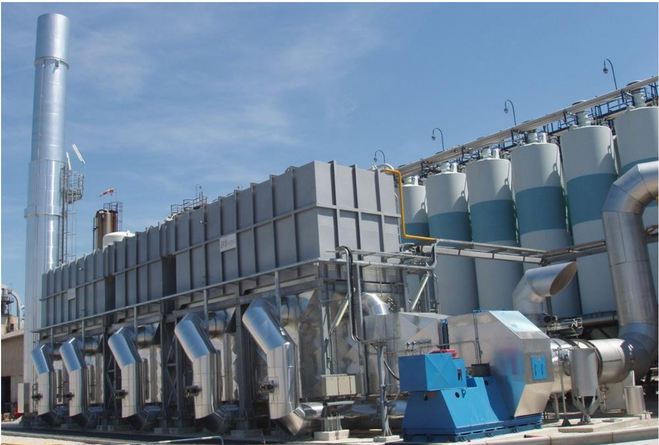
Regenerative thermal oxidation plant.
